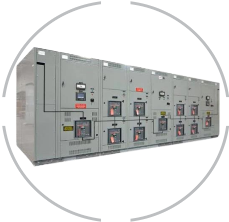
Synchronizing Control Panel
